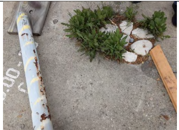
Potential piping associated with USTs (top right)
