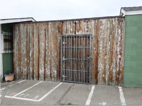
Storage shed with no access
