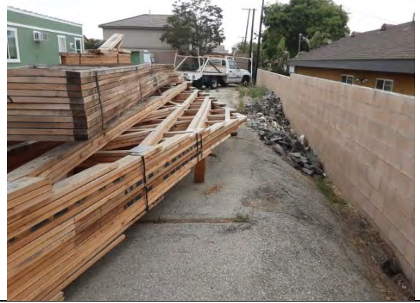
Truss storage and broken concrete
