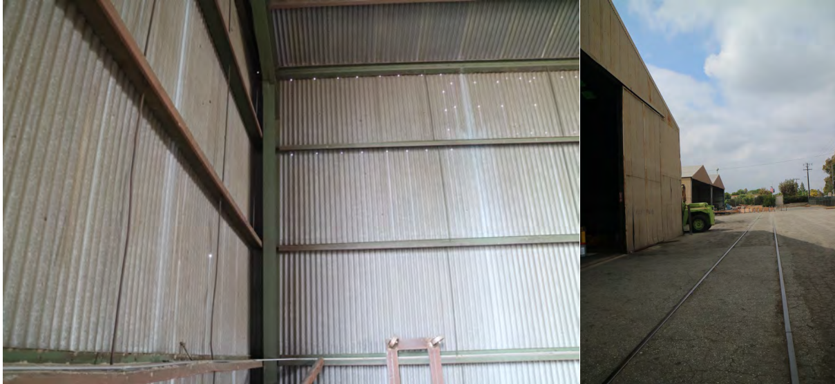
Figure 13. Detail of interior (left, west perspective) and exterior detail with adjacent, decommissioned railway tracks to the north (right, east perspective)
