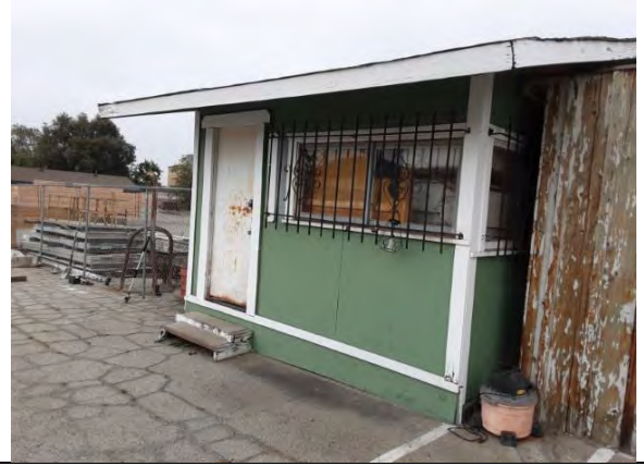
Storage shed with no access
