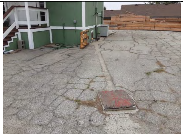
Reportedly associated with electrical utility
